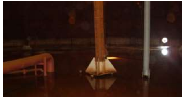
Fig. 6. Detached tank roof support due to irrecoverable bowl-shaped tank raft deformation after hydrotest
