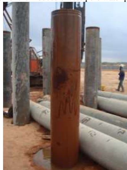
Fig. 1. Water overflowing from inner pile annulus as evidence of high excess pore water pressure within the subsoils in depth
