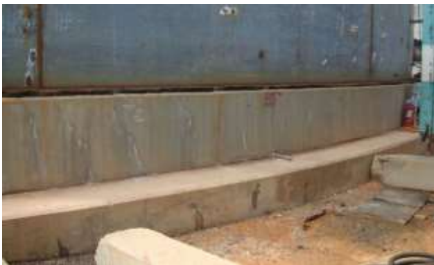
Fig. 5. Tensile cracking on upstand ring beam after hydrotest
