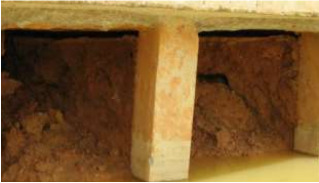
Fig. 2. Settlement of reclaimed platform below tank raft
