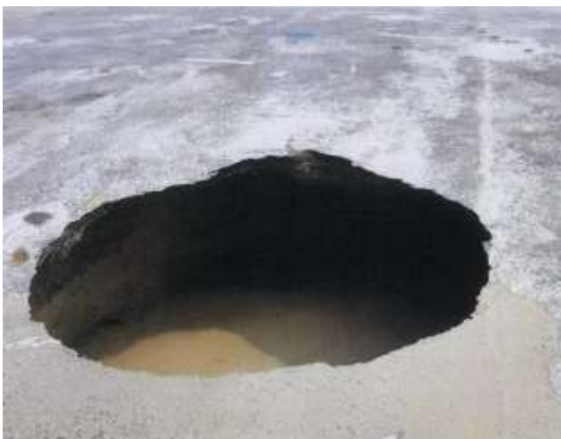
Fig. 8. Typical sinkhole observed on ground surface due to underground construction works in limestone formation.
