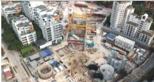
Fig. 5. Overall View of Conlay Station
