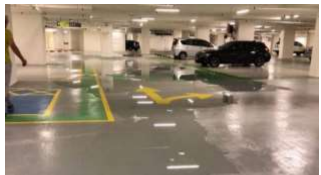
Fig. 5. Spilling of Seepage Water from Collection Drains
