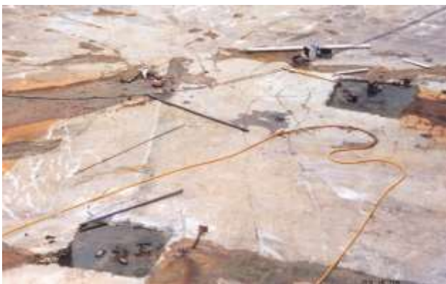
Fig. 2. Flexural Cracks on Open Basement Slab due to Uplift
