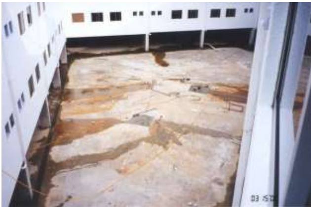
Fig. 1. Overview of Cracked Open Basement Slab with Three Temporary Relief Well Openings
