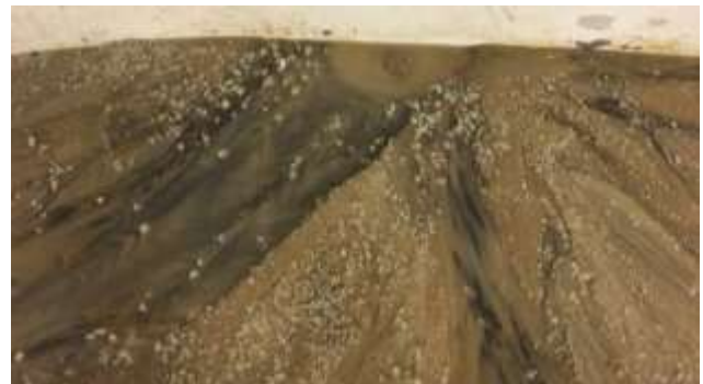
Fig. 4. Washout of Fine Sand in the Seepage through Preferential Flow Path with Piping Erosion Features
