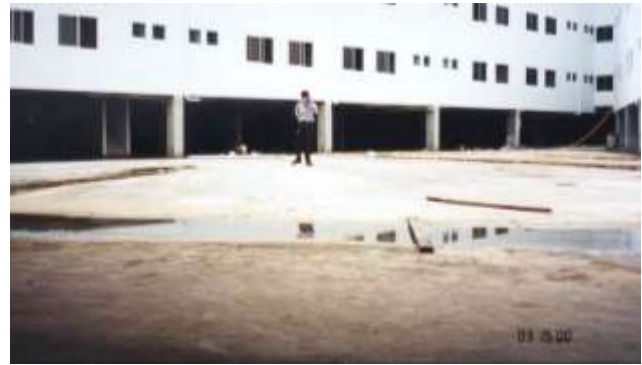
Fig. 3. Maximum Heave of 130mm at Central Portion of Open Basement Slab
