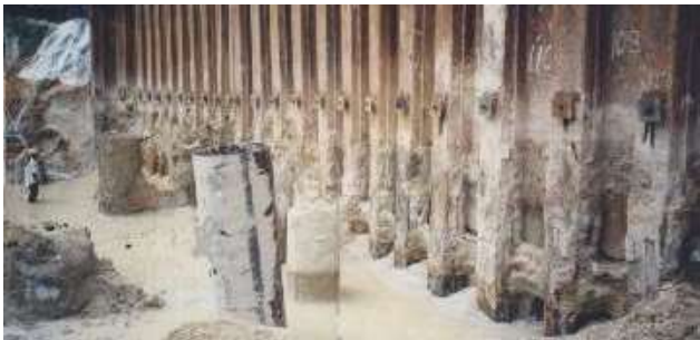
Fig. 11. The Installed Jack-In-Pipe Anchorages at the Sheet Pile Retaining Wall of 9m High
