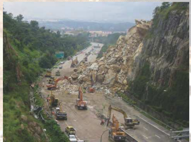
Rock Slope Failure at Bukit Lanjan, 2003
