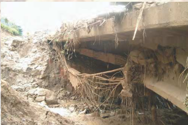
Damaged beam of bridge after hitting by landslide debris
