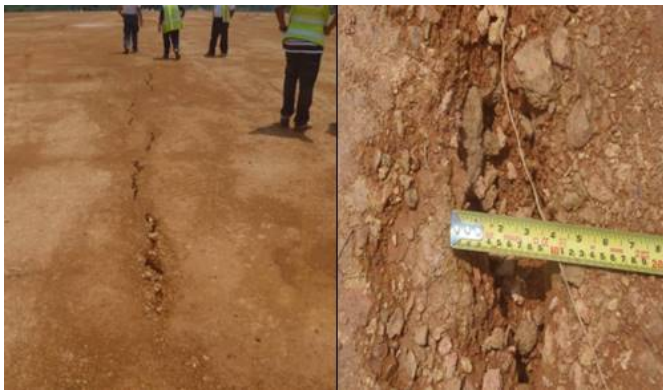
Figure 2 Longitudinal Crack Found at the Embankment
