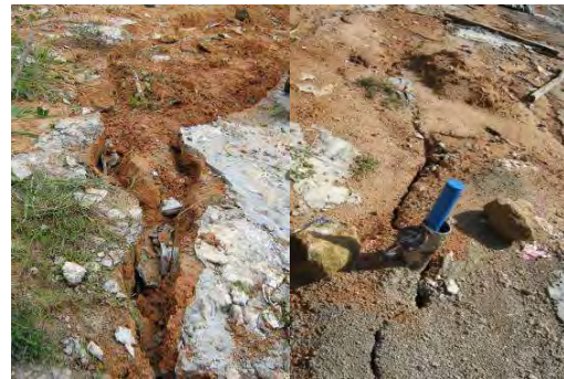
Figure 3 Tension cracks at the crest of the soil nailed slope
