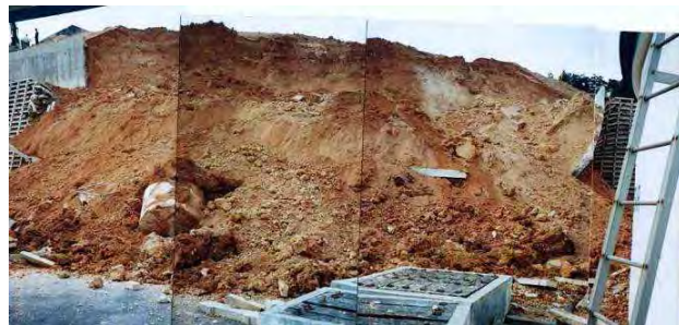
Figure 1 Collapsed Crib Wall and Piled RC Wall
