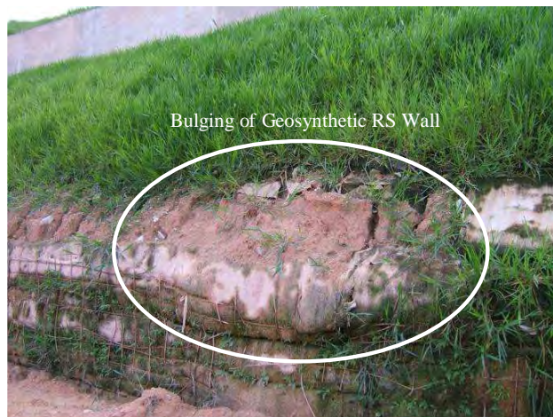
Figure 8 Bulging of Geosynthetic RS wall
