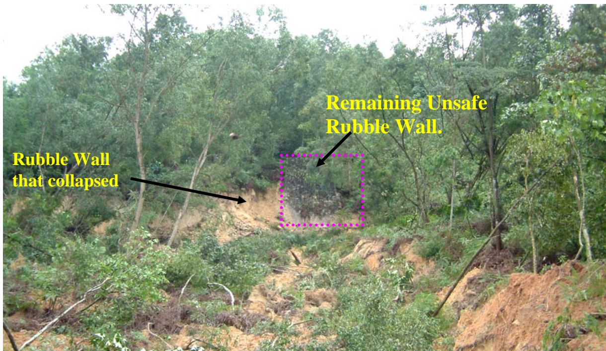
Figure 9 : Close up view of Collapsed Rubble Wall at Taman Hillview failure site.
