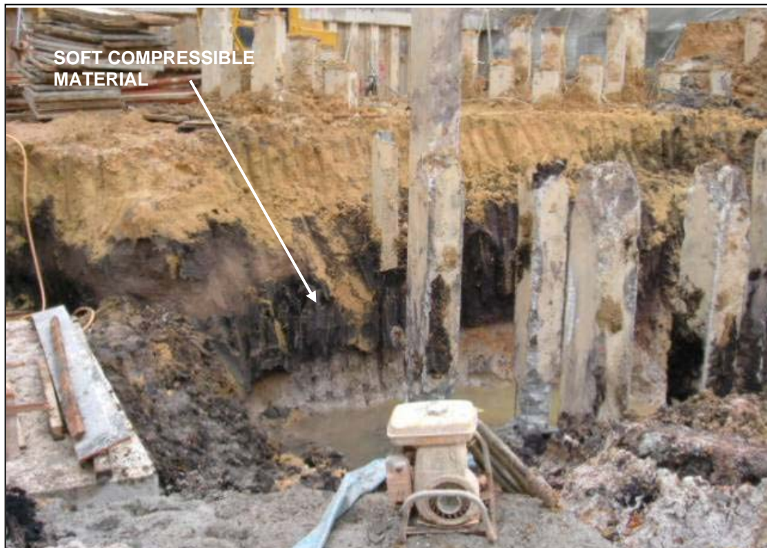
Figure 13: Soft compressible layer detected at localized pile cap excavation
