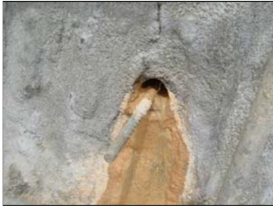
Figure 11: Unset grout and mud slime flowing out during drilling at adjacent nails
