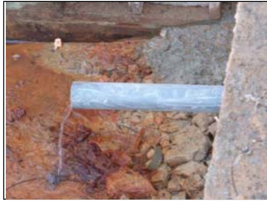
Figure 12: Continuously seepage flow
