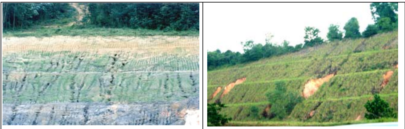
Figure 11: (a) Gullies on Slopes (b) Localised Erosion on Slopes
