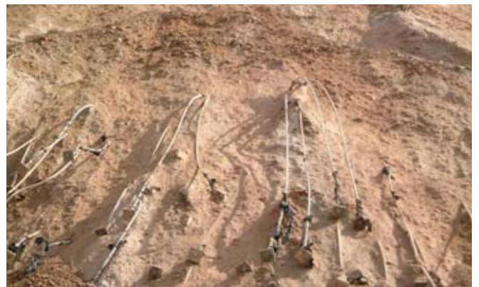
Figure 7. Example of face failure.
