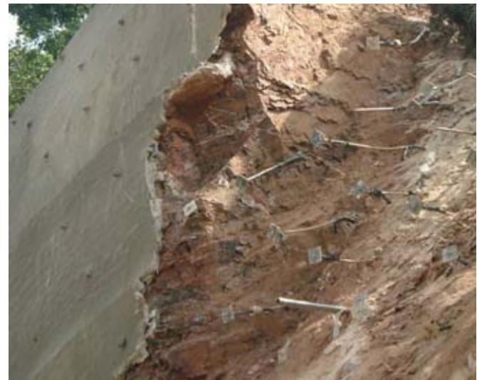
Figure 6. Example of face failure.
