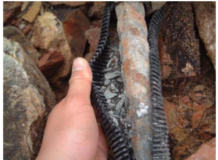
Figure 4. Grout cracked and peeled off from nail – ineffective corrosion protection.
