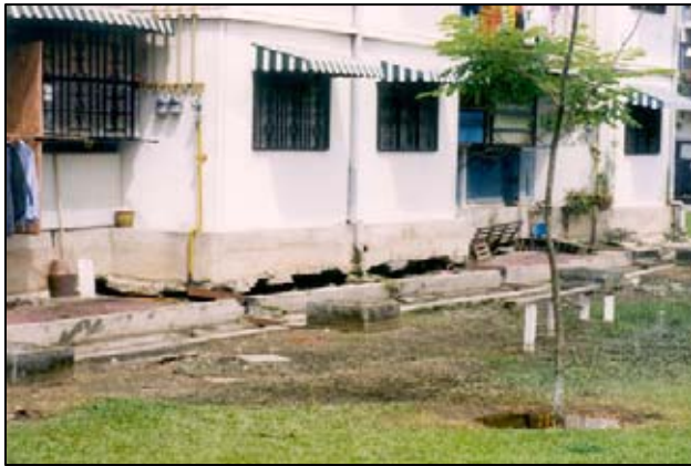
Figure 3 : Settling platform detached from building
