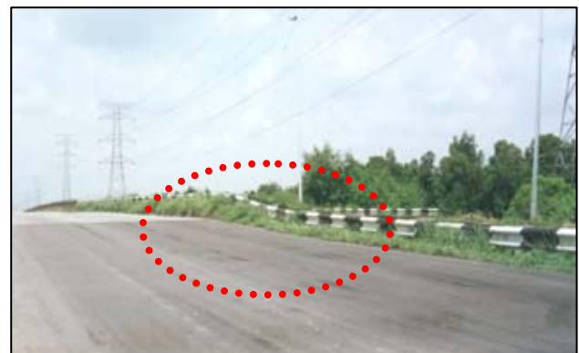
Plate 2 : Hump at Bridge Approach
